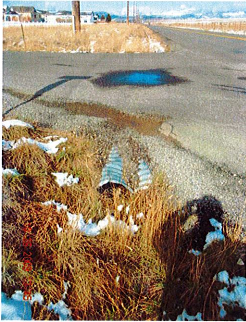
Photo 7: Shallow ditch with a crushed pipe.
