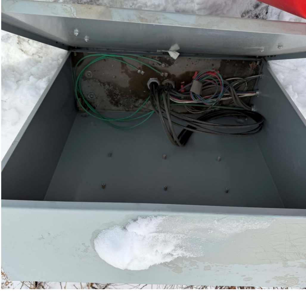
Box between main panel and the generator.
