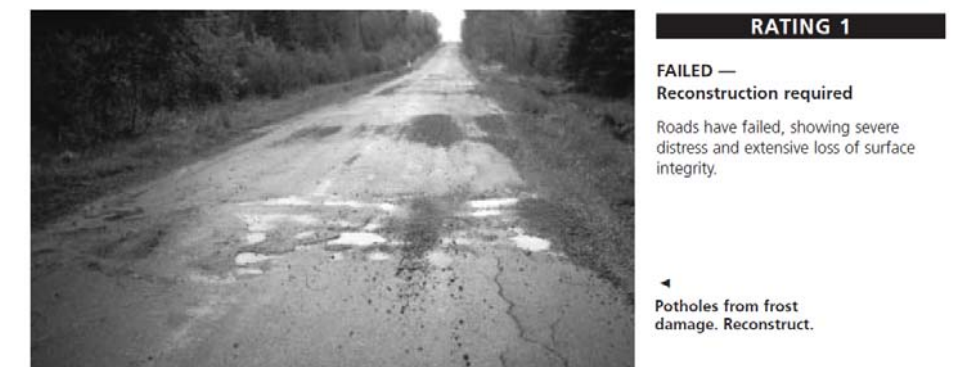
CH 4 FIGURE 2— Poorly constructed and maintained local paved road requires full reconstruction based on the PASER pavement analysis.
