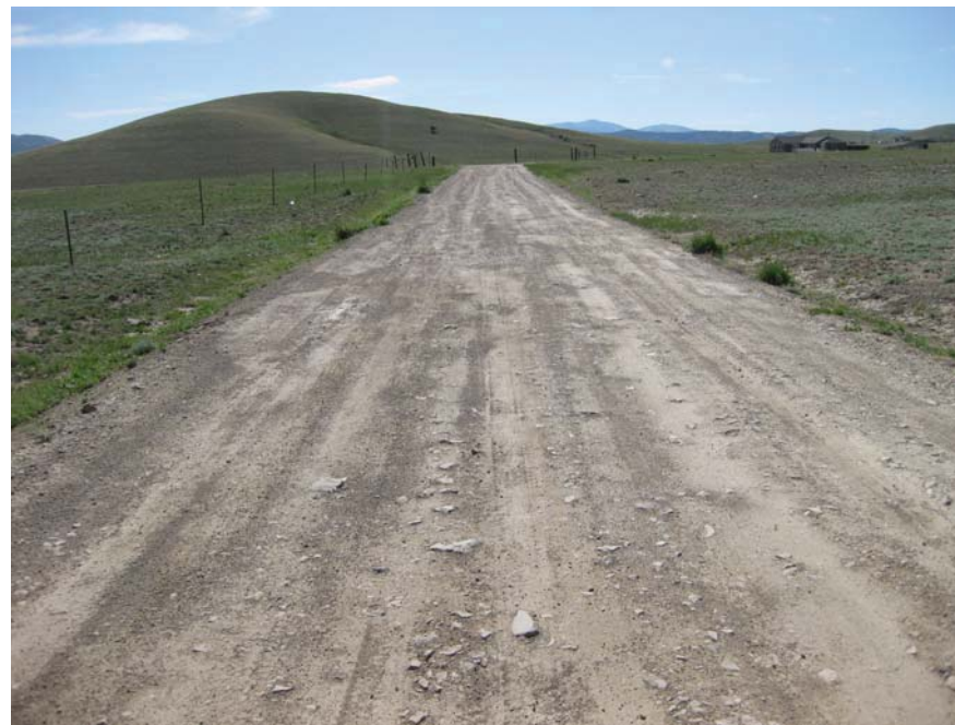
CH 4 FIGURE 1— Poorly constructed and maintained local gravel road proposed to serve a recent subdivision.
