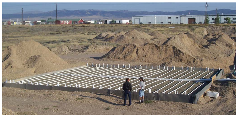
CH 3 FIGURE 1— One of the many private community wastewater systems installed in Helena Valley over the past decade.
